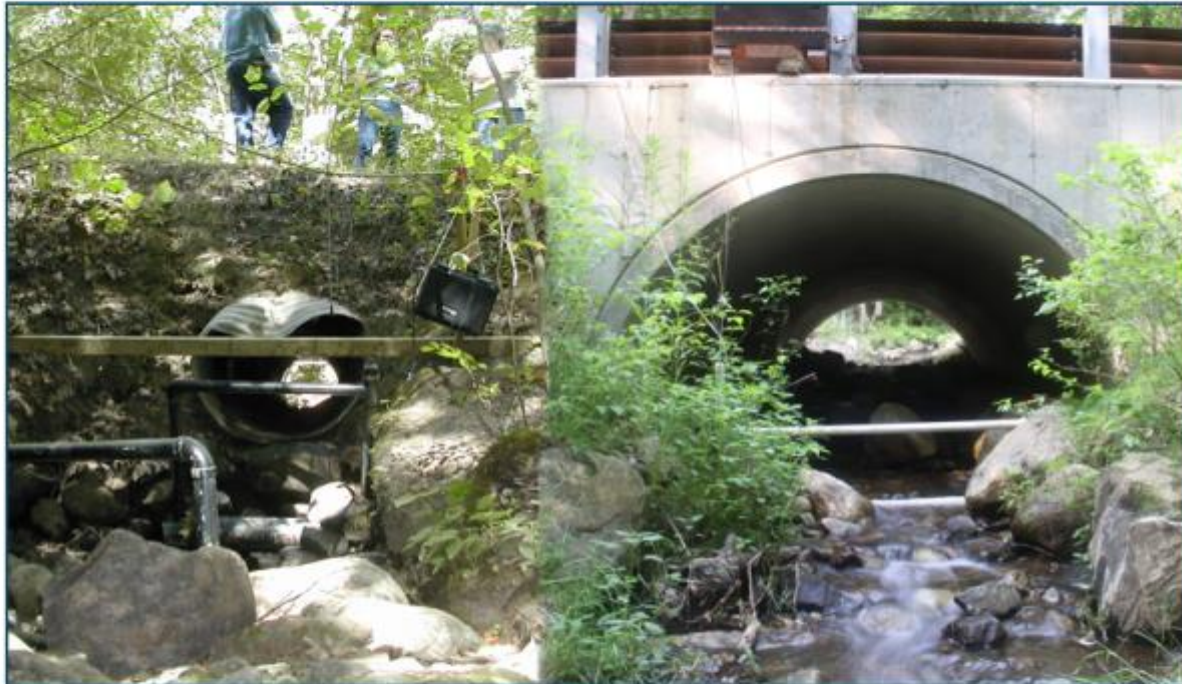
Mitchell Brook in Whately, MA, before and after culvert replacement. The PVC piping in the photos are antennae to monitor the passage of fish through the crossing. Researchers report that not only are more brook trout moving from the West Brook up into Mitchell Brook but dace are now being found in the stream for the first time. Photo credits: Scott Jackson.
